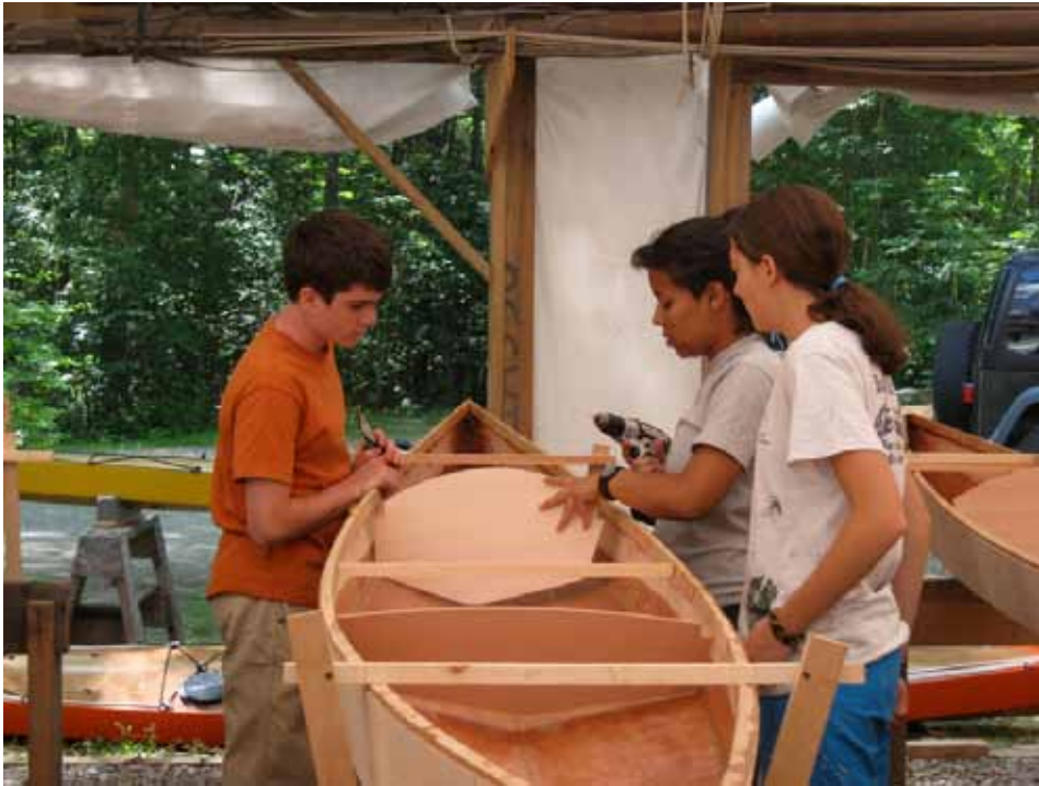
Sam, Chavella, and Nadine find that many hands make bulkhead installation a snap.
