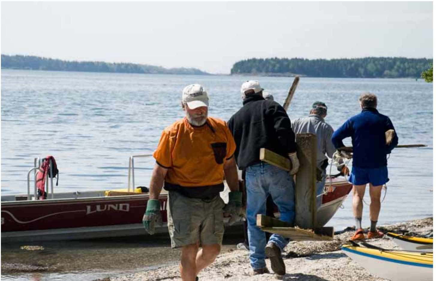
SMSGN volunteers work alongside island owners and MITA staff to dismantle driftwood furniture. Photo by Eliza Ginn
